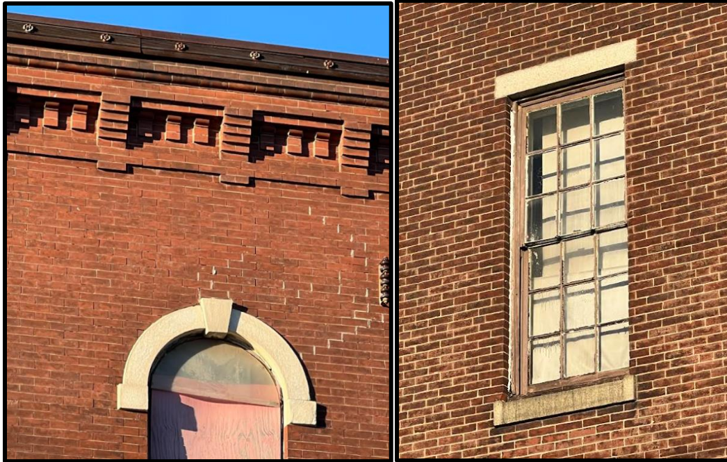
Figure 6a. Left: Window header and cornice detail, Primary (South) Elevation. Figure 6b. Right: An original window, Side (West) Elevation. Source: Oscar Beisert, 2024.
