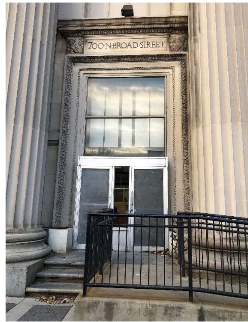
Figure 6. A view of the original main entrance. Original doors have been removed and infilled contemporary doors. An accessibility ramp has been added to the front of the building.
