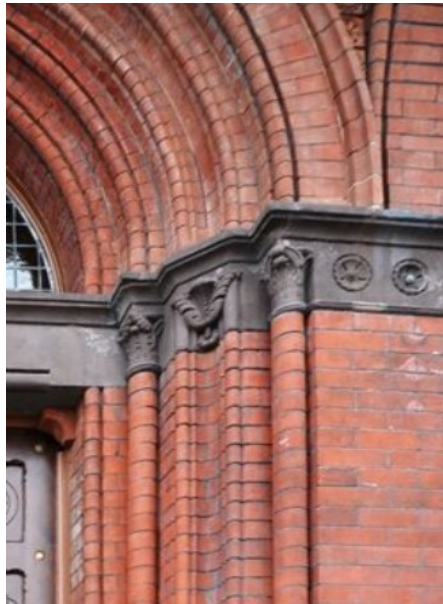
Figure 91: Entrance Detail showing the “rich mouldings of beads, coves, fillets, angles and quirks” created with Peerless bricks.
