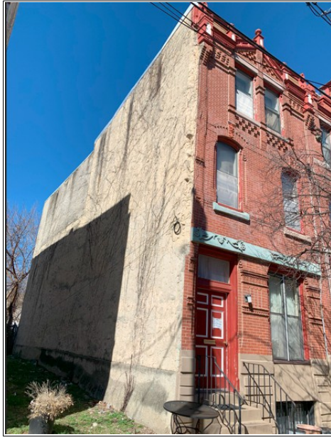
Figure 50: The southwestern wall of 1635 Francis St sits along the property line and was previously a party wall.
