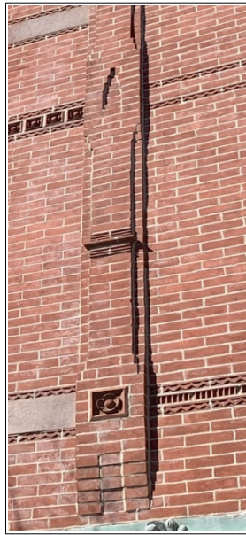
Figure 56: The second-floor "delineator" between 1631 and 1633 Francis St features corbelling at the bottom.
