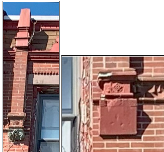
Figures 46 and 47: Two smaller pilasters flank the windows. The left pilaster is relatively intact while the bottom bracket of the one on the right has been replaced by a simpler concrete element.
