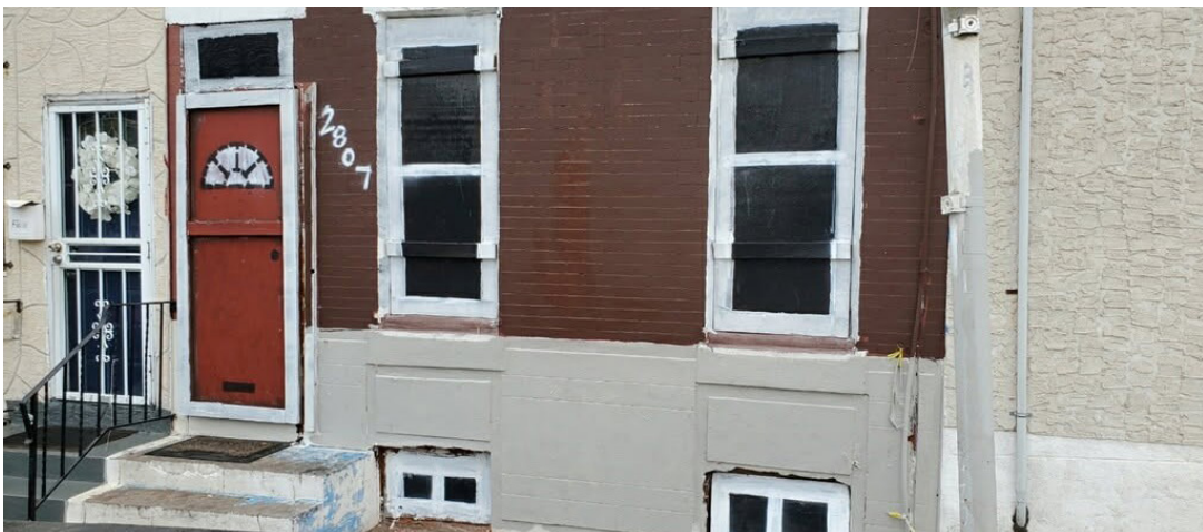
Before and after CLIP's Doors and Windows Initiative, which seals a vacant property and then paints the plywood to resemble doors and windows
