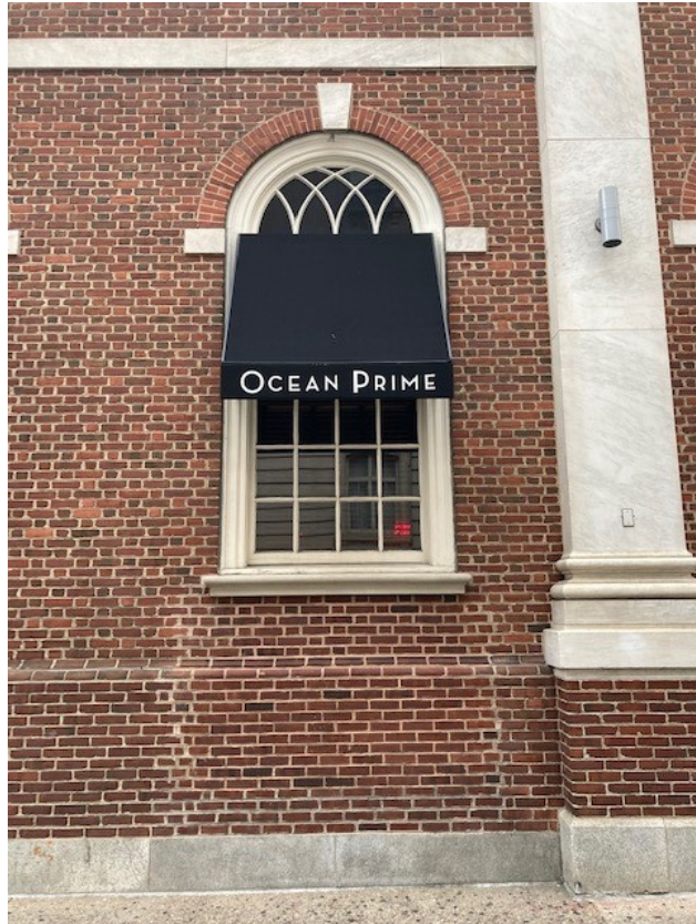
130 S. 15 TH STREET. DETAIL OF CLOSED-UP WINDOW OPENING SHOWING SCARRING FROM REVERSED ENLARGEMENT. PHOTO BY PAUL STEINKE, 8/17/21.
