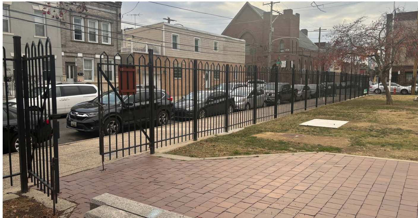
Existing perimeter fence & gates non-compliant (infill spaced wider than 4"); remove and replace with compliant alternative
