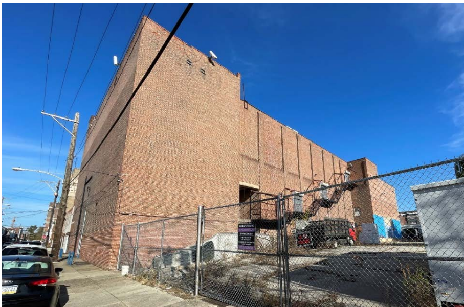
Figure 16: South elevation of subject property, viewed from Carlisle Street. The uneven gray portion at the base of the rear side wall appears to be a remnant of a wall on the adjoining parcel.
