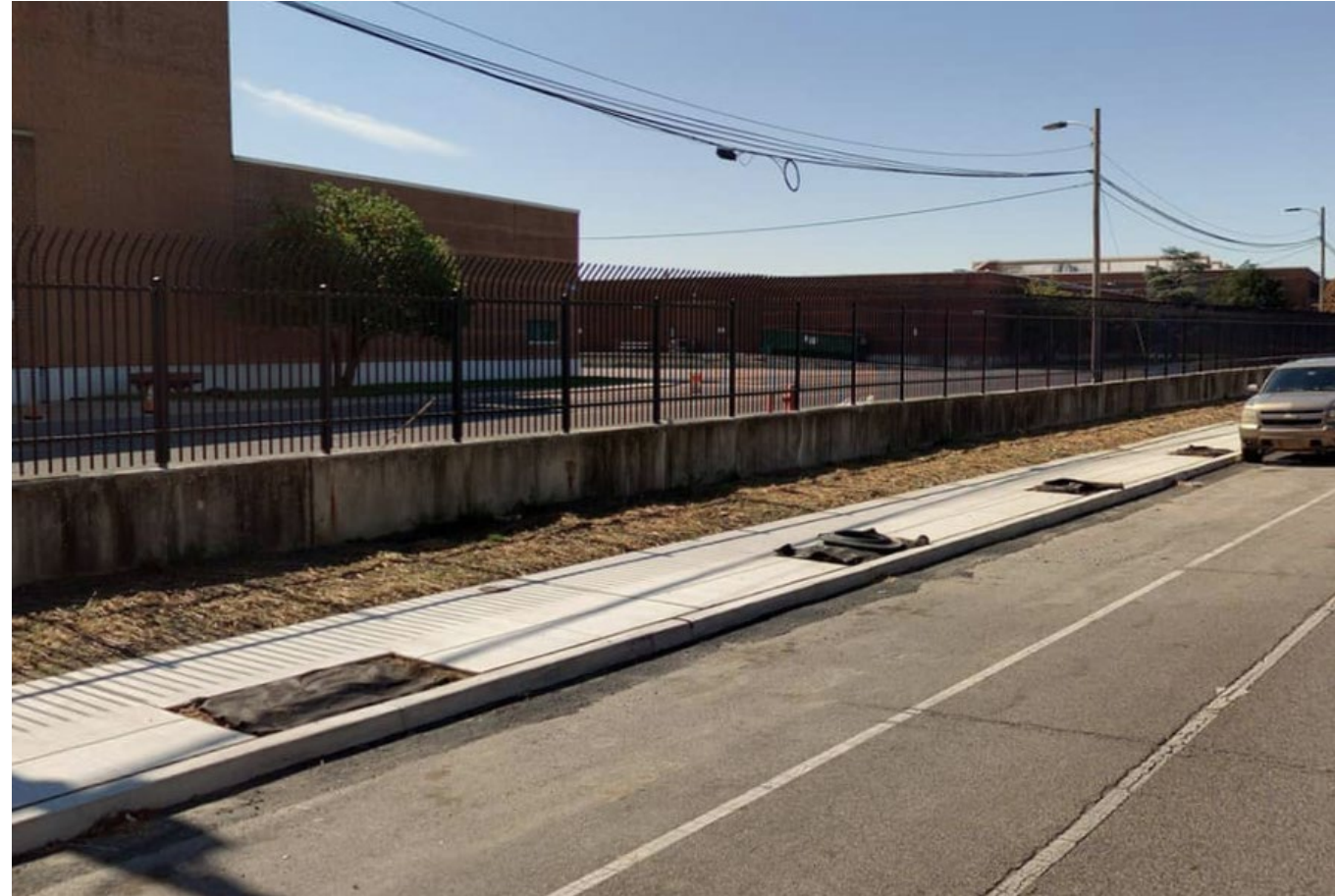
PWD is installing tree trenches and tree pits as part of its GSI project
