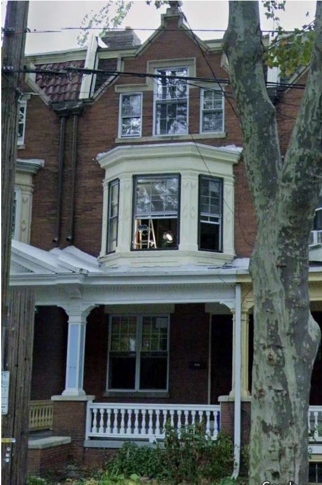
Figure 2. 327 N 34 th Street, 2024. Front façade showing vinyl replacement windows. Image source: Google Streetview.
