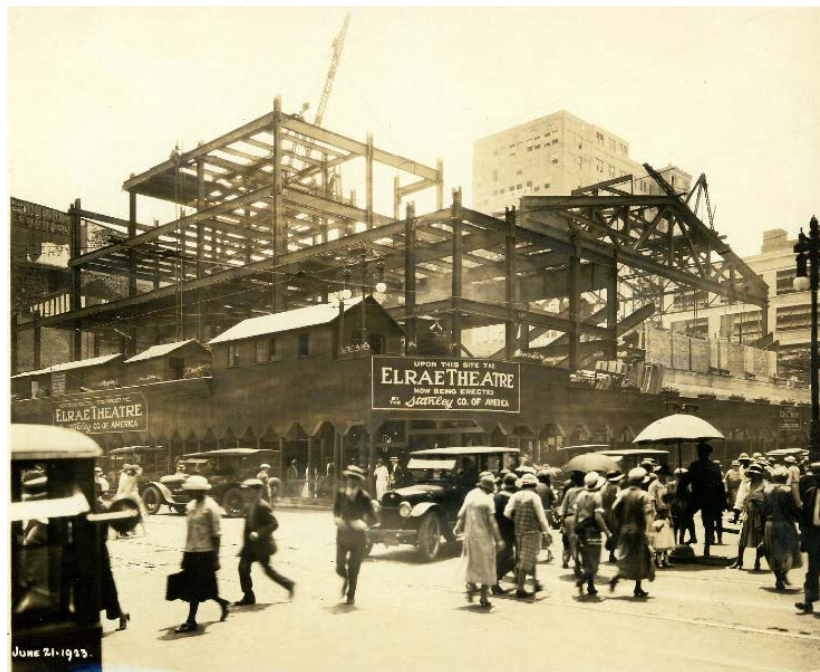
Figure 32: Photo of the Earle Theatre (then called the Elrae) under construction shows the steel skeleton under the masonry façades. Photo from the Glazer Theater Collection.
