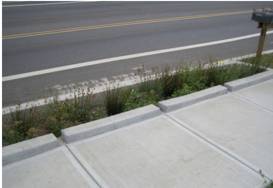
Curb inlets allow stormwater to flow into planter strips.
