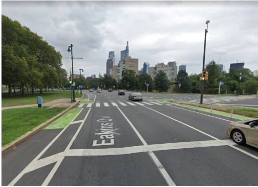
Green colored pavement at the intersection of Eakins Oval and Spring Garden Street
