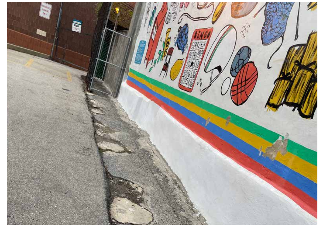
Existing asphalt to be demolished and be converted to ages 2-5 play area.
