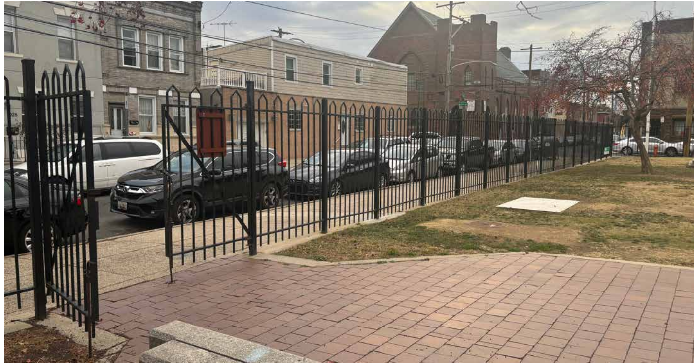
Existing perimeter fence & gates non-compliant (infill spaced wider than 4"); remove and replace with compliant alternative
