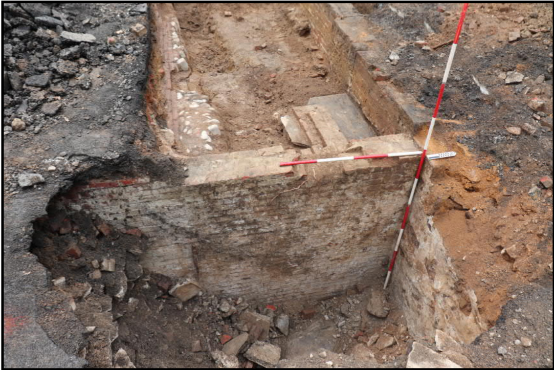
Photograph 3.13. View facing northwest showing the brick and brownstone walls of the Wharton Public School basement (Photographer: Michael Brown, July 2019) [HRI Neg.# 19027/D1:272].
