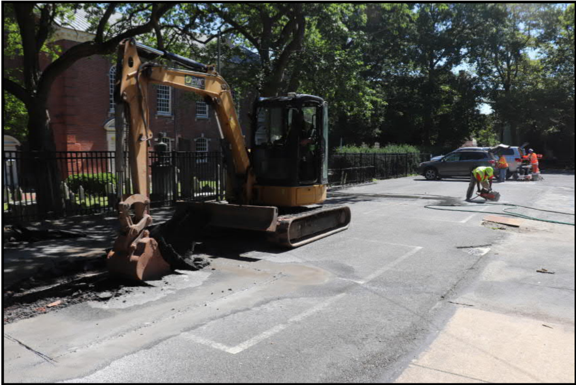
Photograph 3.1. View facing northeast showing the mechanical stripping of Test Pit A. At the mid-point of the frame the asphalt overlying Trench 1 is being cut with a road saw (Photographer: Andrew Martin, July 2019) [HRI Neg.# 19027/D1:034].
