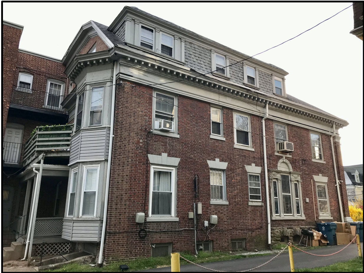
Figure 8. Northeast elevation taken from the rear, or south side, of the property at 150 W. Washington Lane illustrating its connection to a later addition and modifications. Source: Keeping Society of Philadelphia, 2023.
