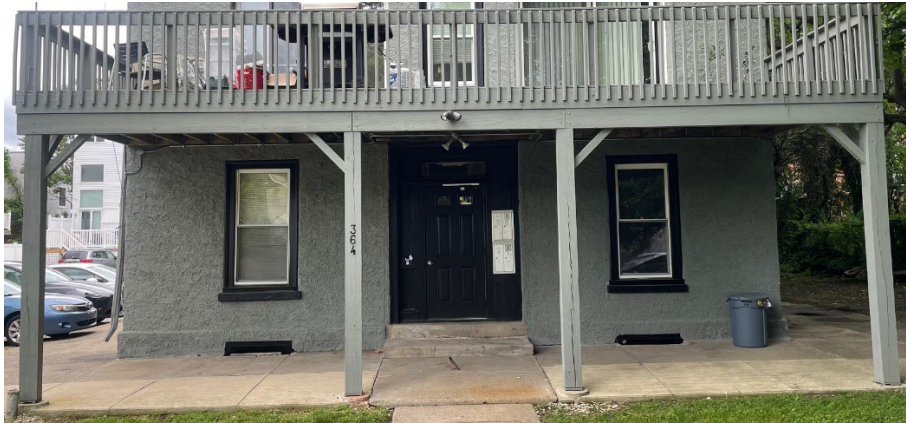
Fig. 7. Lower front façade with differing pavements indicating changes to the lower facade >The front deck has the architectural character of the wild west – no ornament of the period; the paving makes clear that for some period of time there was no porch.
