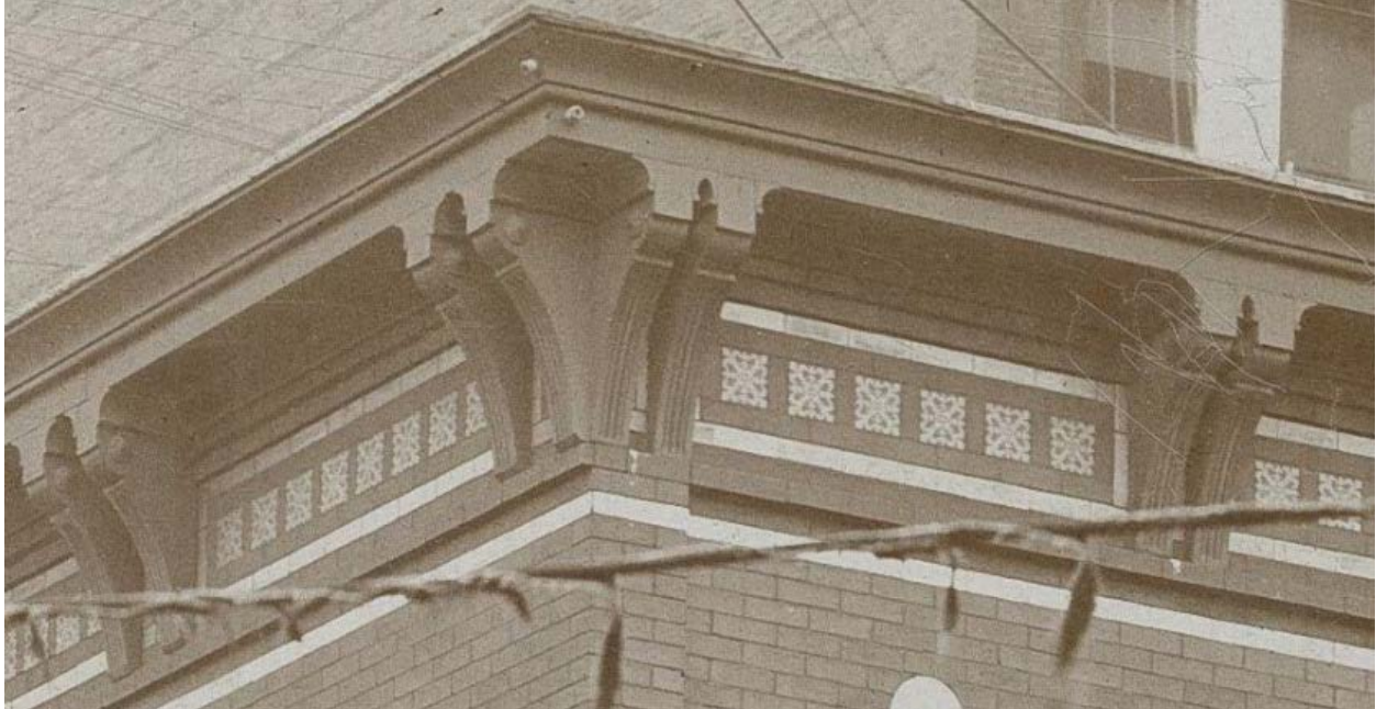
Figure 36: Detail from a turn-of-the-century photograph shows the ornament and cornice before the façade was painted.
