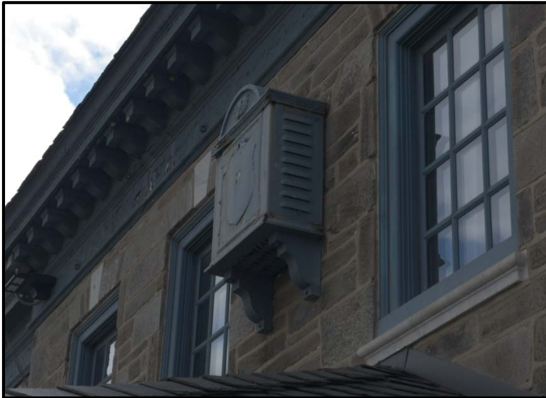
Figure 10. An early alarm device on the Chestnut Hill Office of the Germantown Trust Company, 8527-29 Germantown Avenue, Rear (Northeast) Elevation. Source: Oscar Beisert, 2024.
