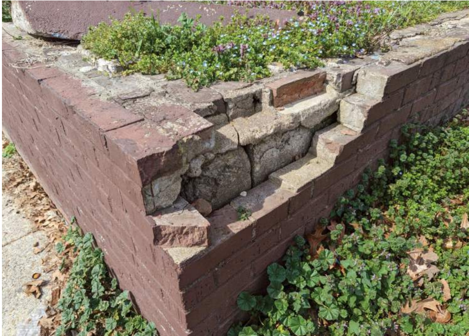
FIGURE 3: CRUMBLING RETAINING WALL
