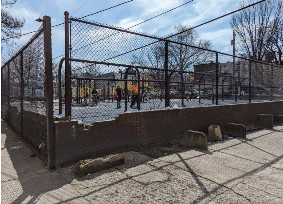
FIGURE 4: CRUMBLING WALL AND FENCE
