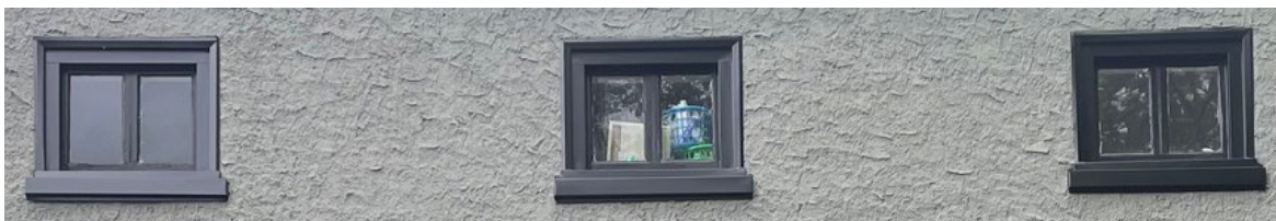
Fig. 8. All of the third-floor sash are modern in configuration; the frames are modern as well; and the group exists in a sea of modern wavy stucco.
