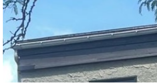
Front cornice reduced to single plank
