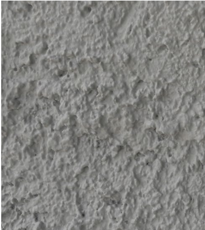
Fig. 9. Gloppy, sprayed on painted, non-historic stucco surface
