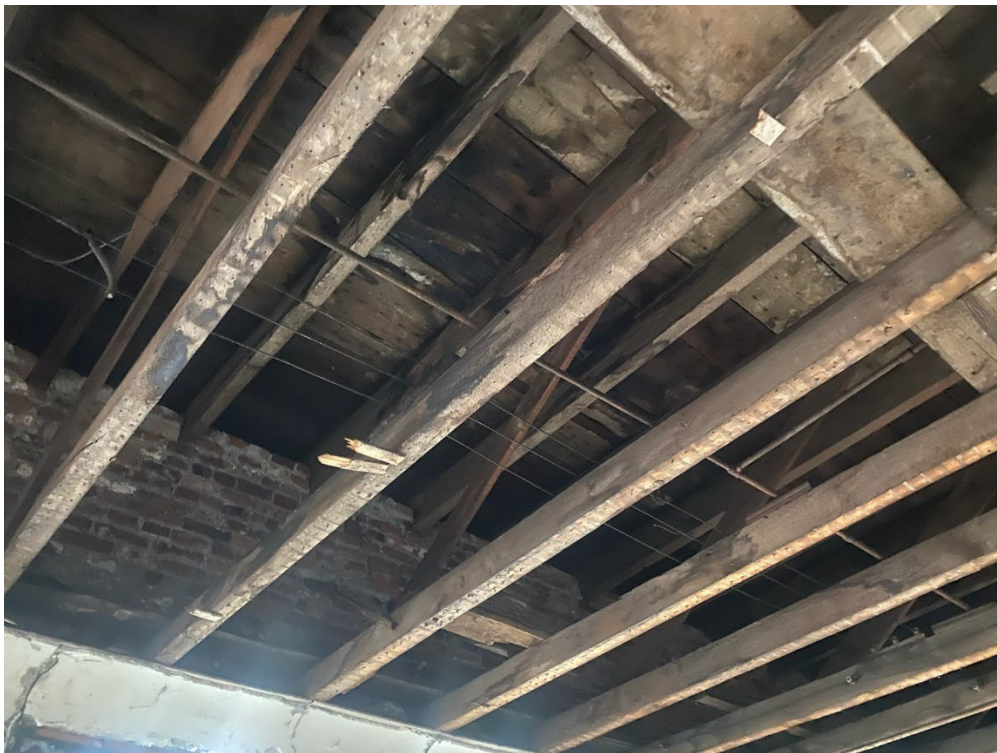
Rotted roof planking, rotted roof planks, removed finishes from water damage
