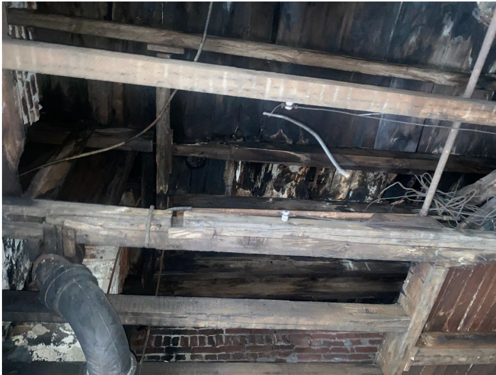
Black rot on roof planking, upper floor; evidence of systemic water damage throughout
