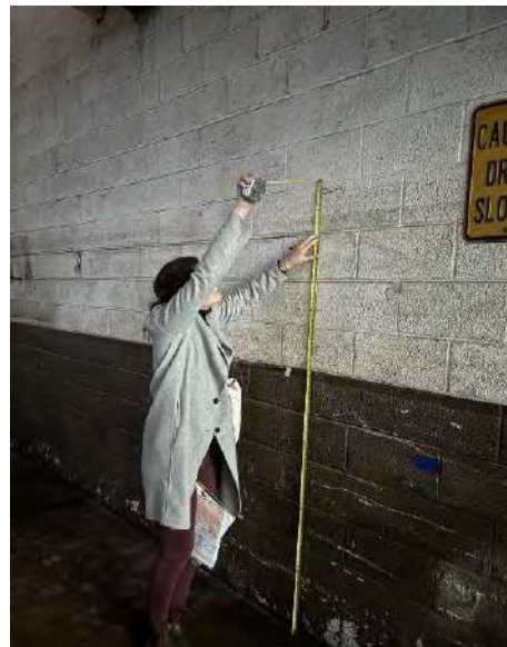
Figure 6: Highwater mark within the building for Hurricane Ida (2021).
