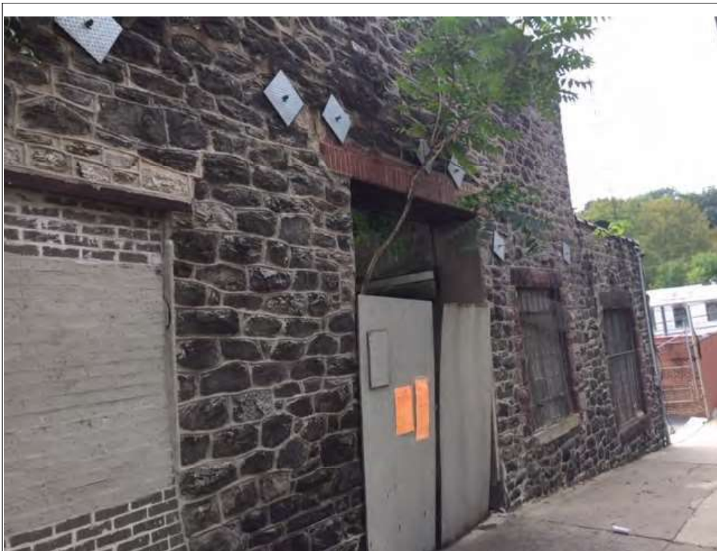
Current decaying facade
