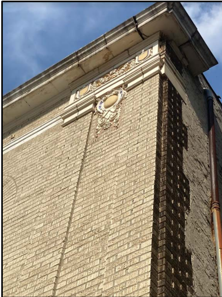
Figure 8. Architectural terracotta details and tapestry brick within the primary (west) elevation. Source: Andy Molholt, 2024.
