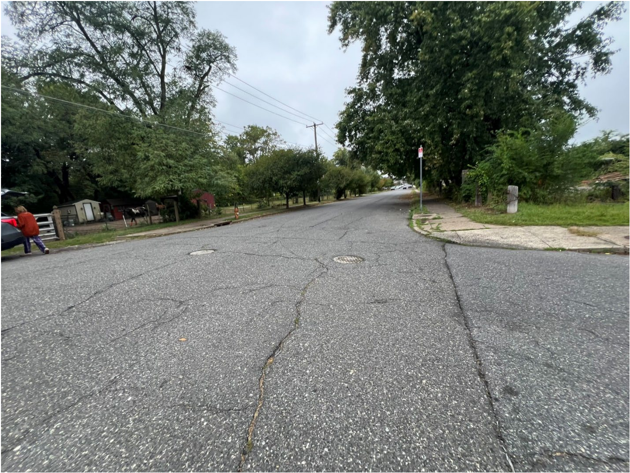
View looking West of 8121 Verree Road from Solly Avenue at Rising Sun Avenue
