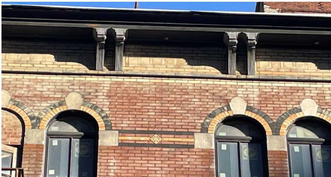
Figure 39: Detail showing the fourth-floor ornament as well as the cornice, which features a band of tiles as well as several courses of colored bricks. This elevation was previously painted, obscuring some of the flourishes.
