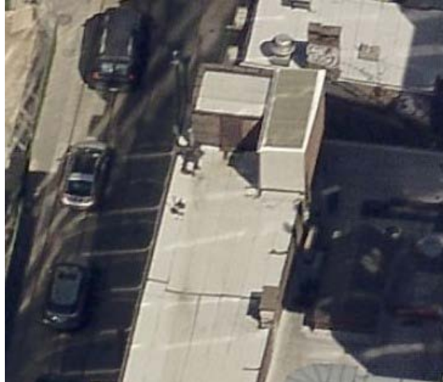
Figure 16: Aerial view of the utility room/pilot house on the roof of 1039 Chestnut Street and the party wall with 1037 Chestnut Street (right). Image from Pictometry.phila.gov.
