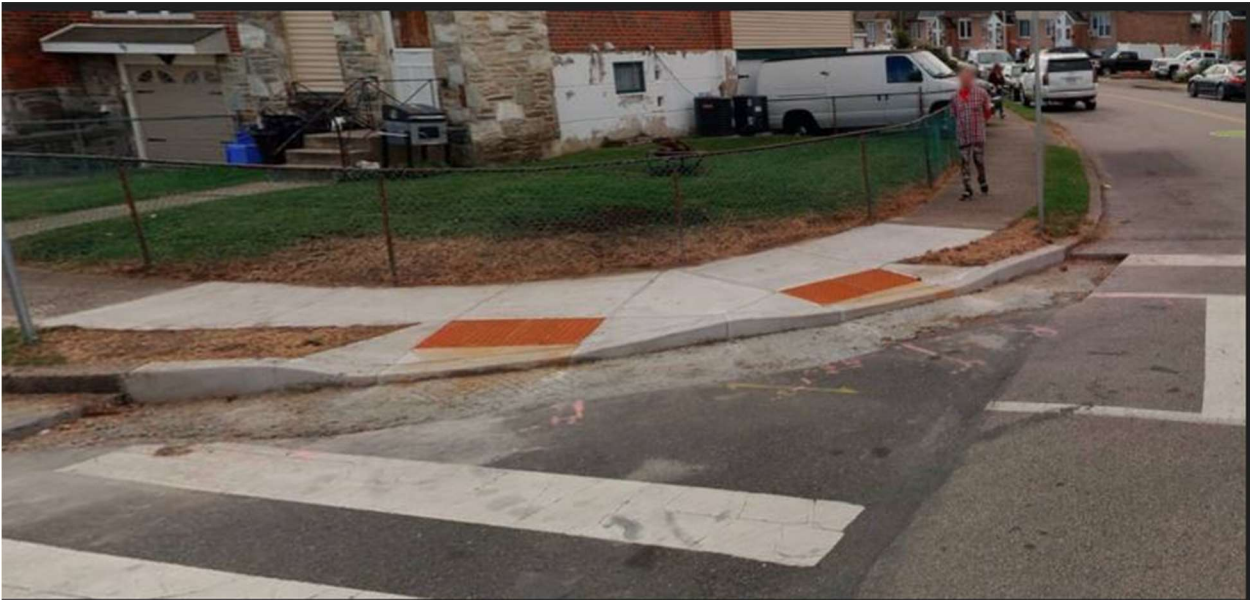
Before and After of Compliant ADA Curb Ramp at Drumore Drive and Modena Drive
