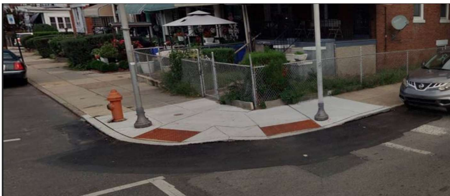
Before and After of Compliant ADA Curb Ramp at 57 th Street and Larchwood Avenue
