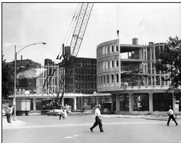
Figure 8: Circa 1960 photograph of the construction of the Philadelphia Police Headquarters. (Source: Urban Archives, Temple University)
