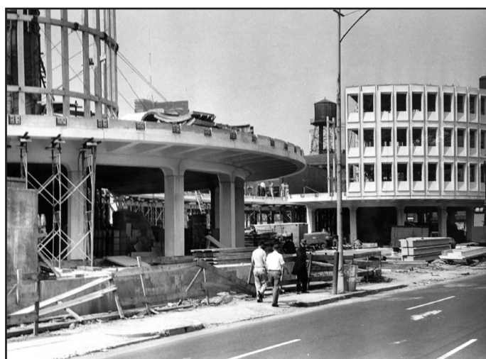
Figure 9: Circa 1960 photograph of the construction of the Philadelphia Police Headquarters. (Source: Urban Archives, Temple University)
