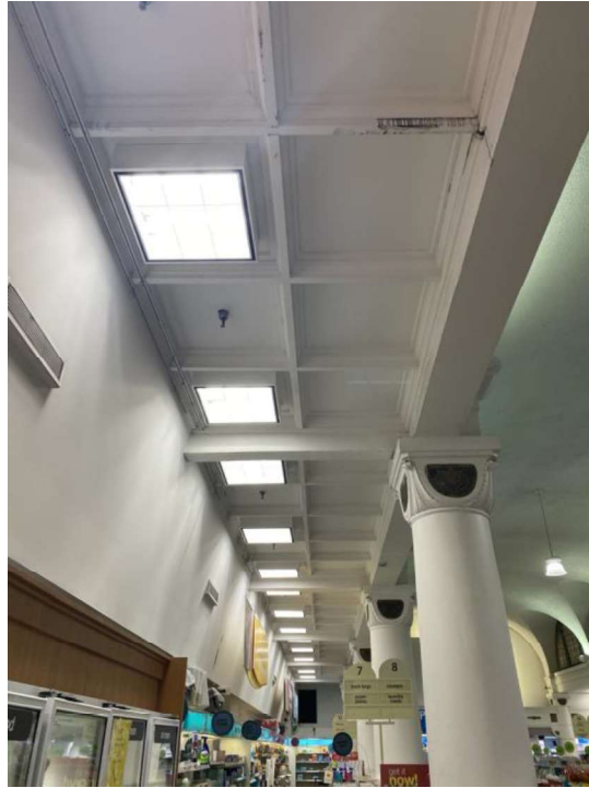
Figure 16 – Typical side aisle skylights (October 2021). At far left, a drywall bulkhead conceals a third row of skylight panels, a condition which is mirrored on the opposite side of the space.
