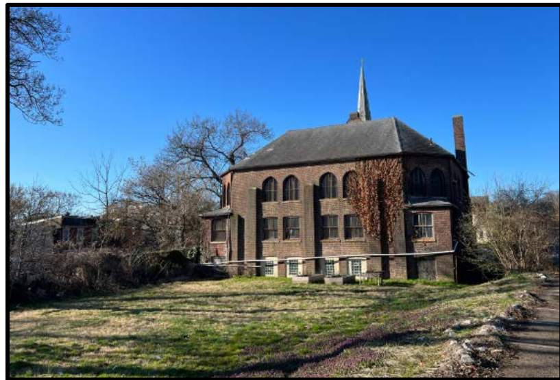
Figure 11. Top: The primary (southwest) elevation of the 1916 Addition to St. Stephen's M. E. Church. Source: Oscar Beisert, 2023. Figure 12. Bottom: The rear (northeast) elevation of the 1916 Addition to St. Stephen's M. E. Church. Source: Oscar Beisert, 2023.
