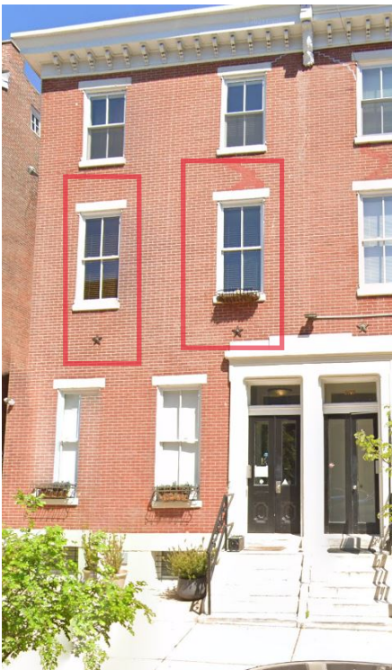
1615 GREEN ST., APT. B 2 WINDOWS PROPOSED FOR IN-KIND REPLACEMENT MARKED IN RED
