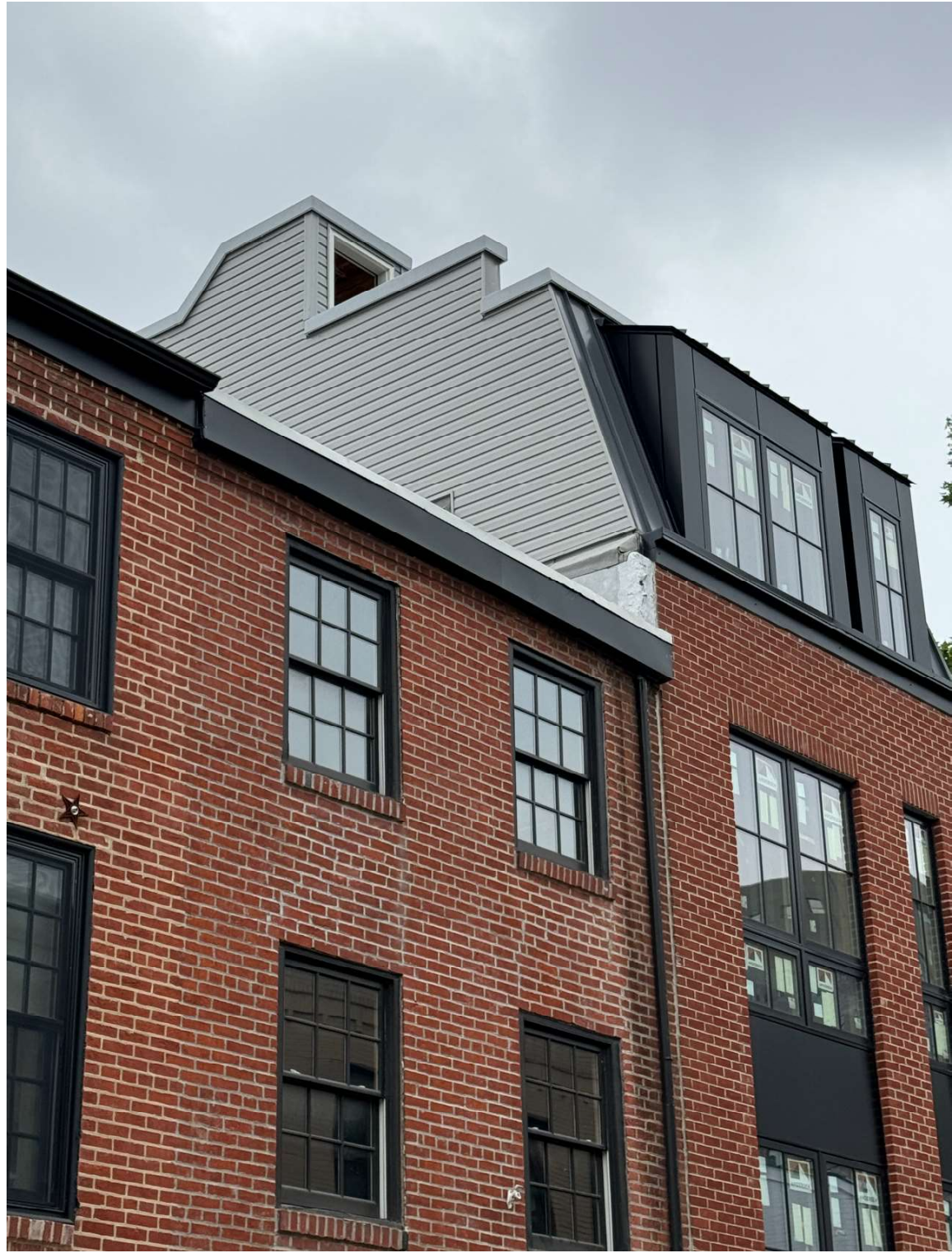
Figure 4. 1930 Pine Street rear along Waverly Street, showing visibility of pilot house clad in vinyl siding. July 2024.
