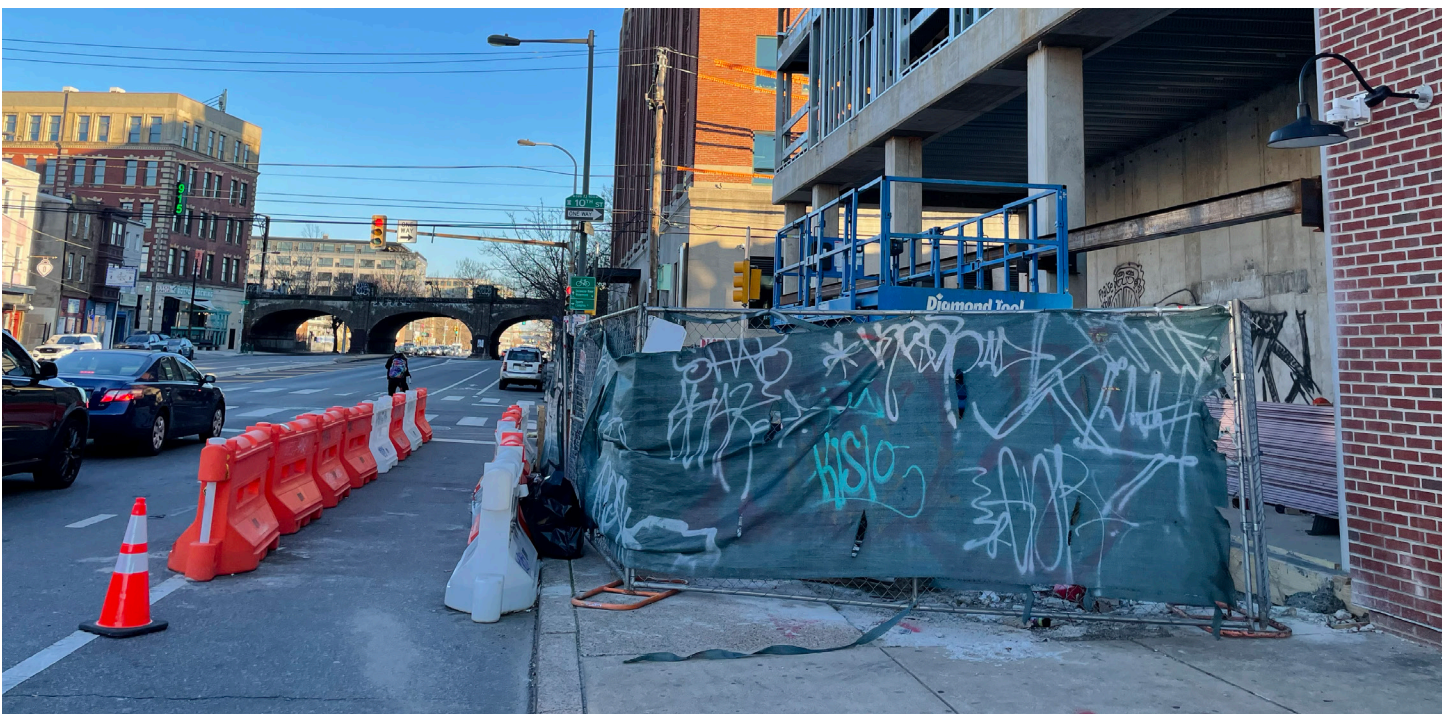
Sidewalk closure due to construction on the corner of Spring Garden and 10th Streets facing east, Source: Sojourner Consulting
