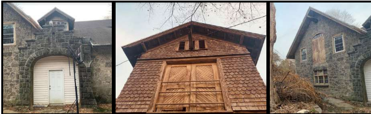
Figure 69. Left: A alteration to the central vehicle entrance of the primary (northwest) elevation of the Carriage House & Stable. Figure 70. Center: A projecting loading dormer on the second floor of the side (southwest) elevation, featuring much of its original details. Figure 71. Right: The northeastern most component of the primary (northwest) elevation of the Carriage House & Stable. Source: Oscar Beisert, 2019.
