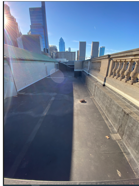
VIEW FROM UPPER ROOF, FACING SOUTH. THERE IS NO EXISTING MECHANICAL EQUIPMENT.
