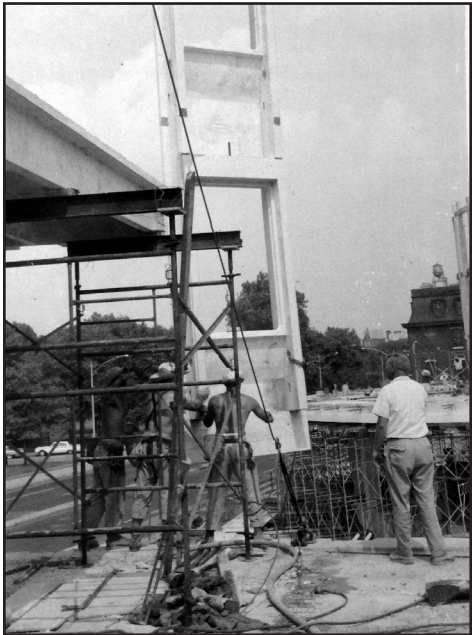
Figure 10: Circa 1960 photograph of the construction of the Philadelphia Police Headquarters. (Source: Architectural Archives, University of Pennsylvania)
