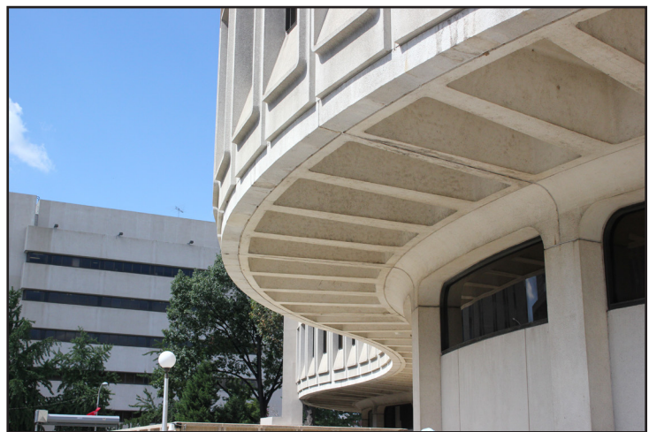
Figure 5: View of the underside of the cantilevering upper floors (Source: Allee Davis, September 2012)
