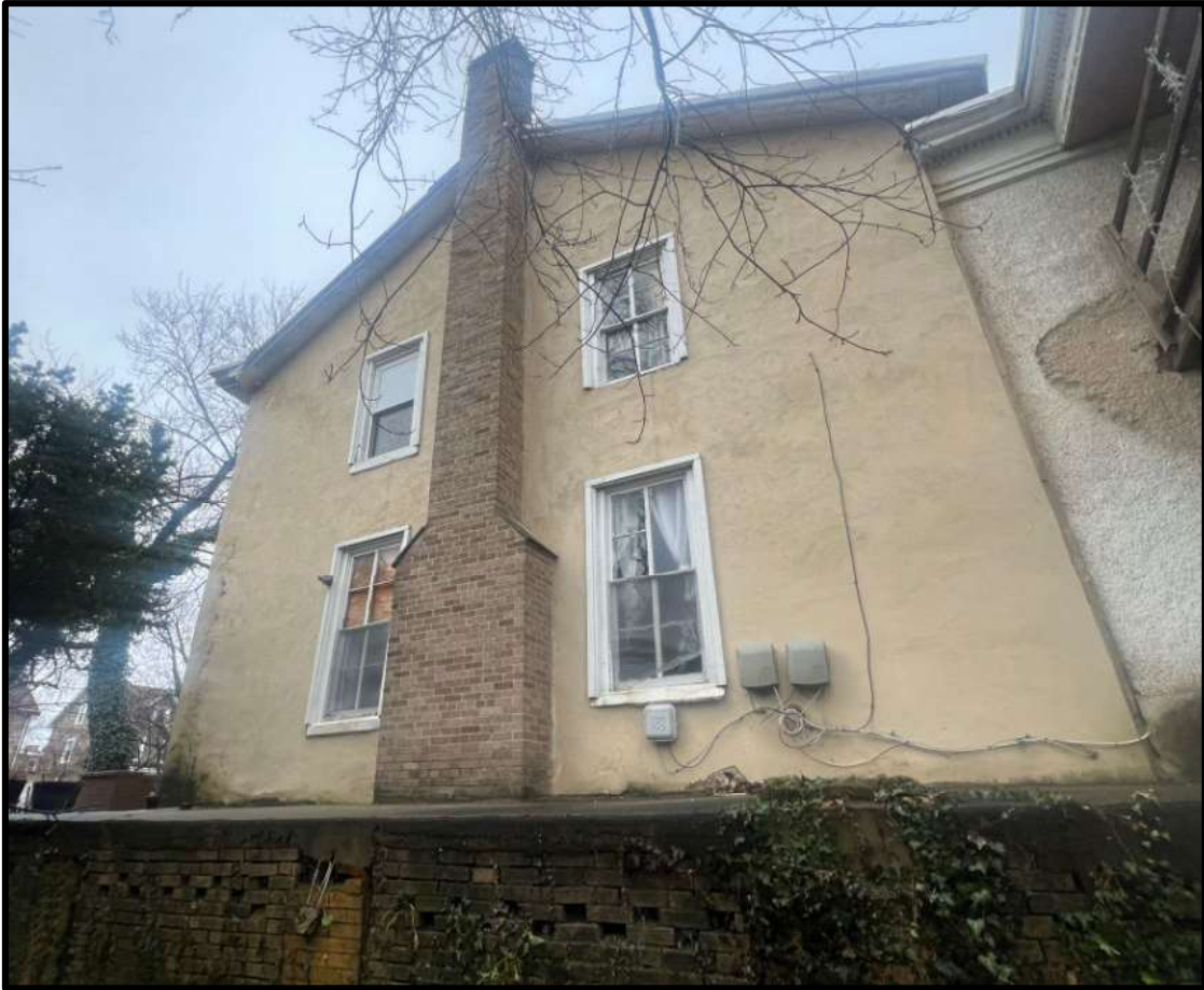
Figure 10. The Smith-Steel-Humphreys House, 424 E. Woodlawn Street, Side (Southwest) Elevation of the Main Block. Source: Oscar Beisert, 2023.
