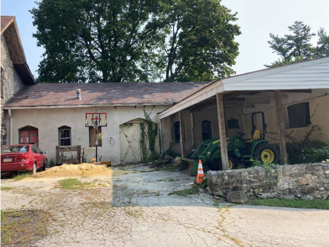
Figure 18: September 2022 photograph showing the existing conditions of the stable. View looking east.
