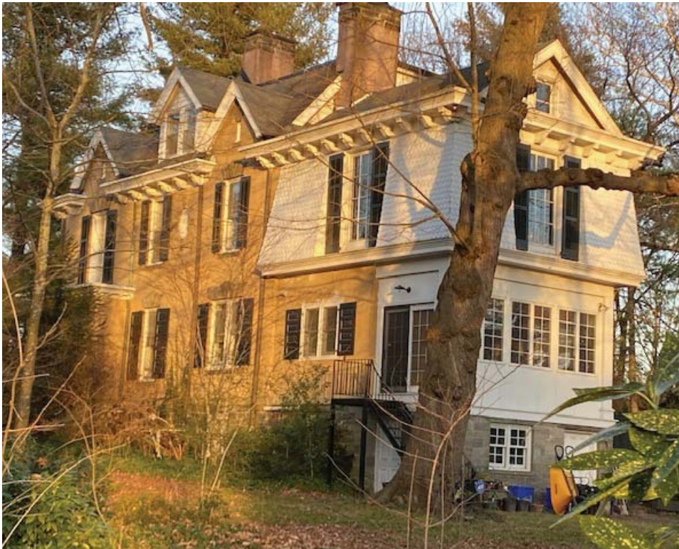
Figure 7. Back of the northwest facade of The Yellowstone. Chestnut Hill Conservancy, January 2022.
