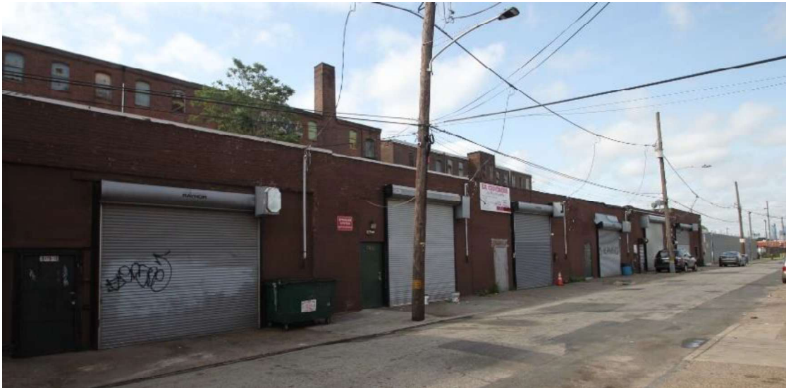
Figure 18: West elevation of the Garage building, view southeast. As shown in Figure 17, this elevation once contained smaller openings with windows rather than the garage doors that exist today (the doors were likely installed after 1950).
