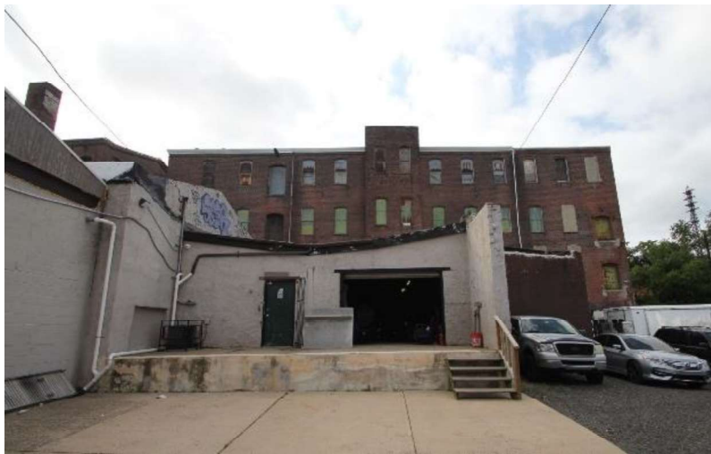
Figure 14: West elevation of Mill #2, view east. The one-story, concrete block structure with loading dock in the foreground is part of the post-1950s additions.
