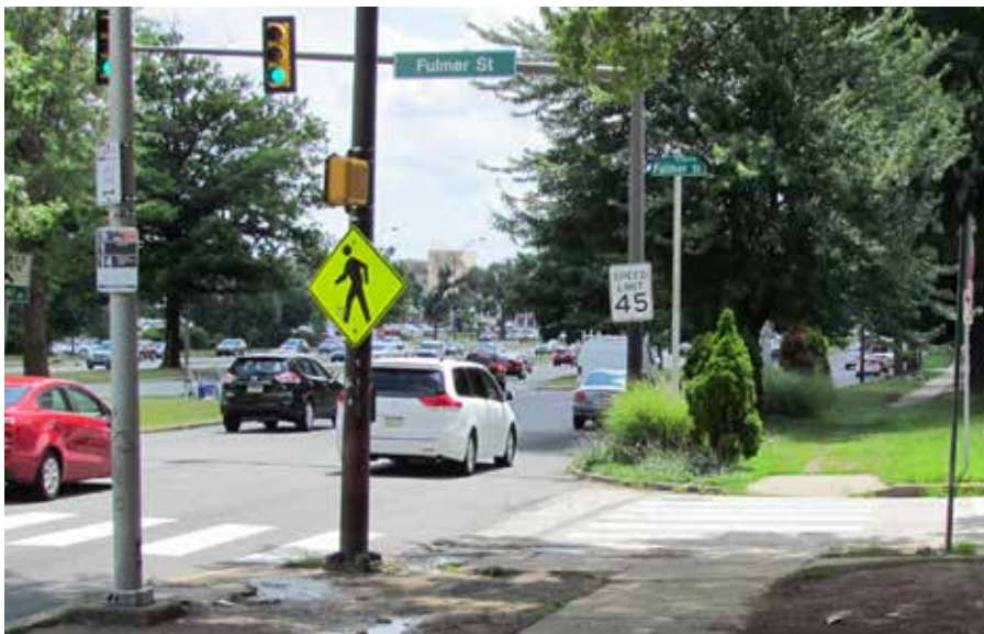
Figure 8-7. Example of Poor Condition Sidewalk Along the Boulevard
