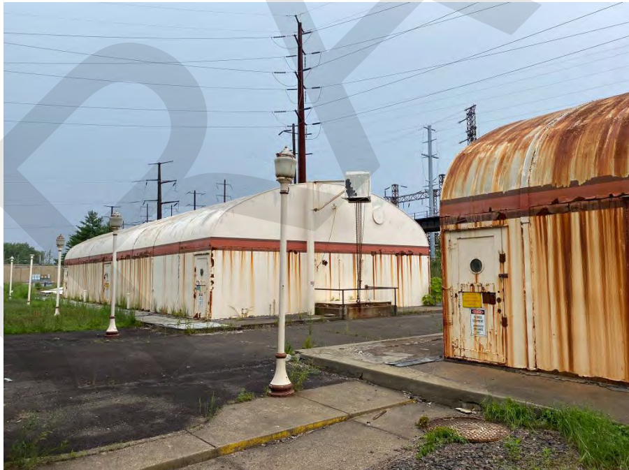
Photo 30 - Converter Unit #3, looking northwest.
