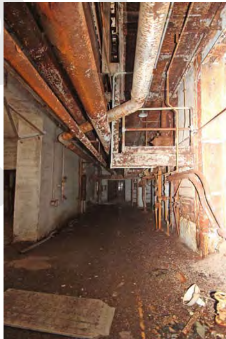
Photo 12 - Boiler House interior, typical boiler equipment.
