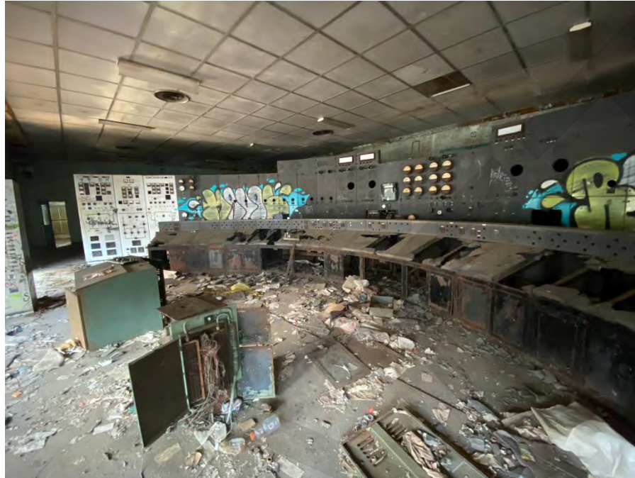
Photo 19 -Control Room on fourth floor, looking south.
