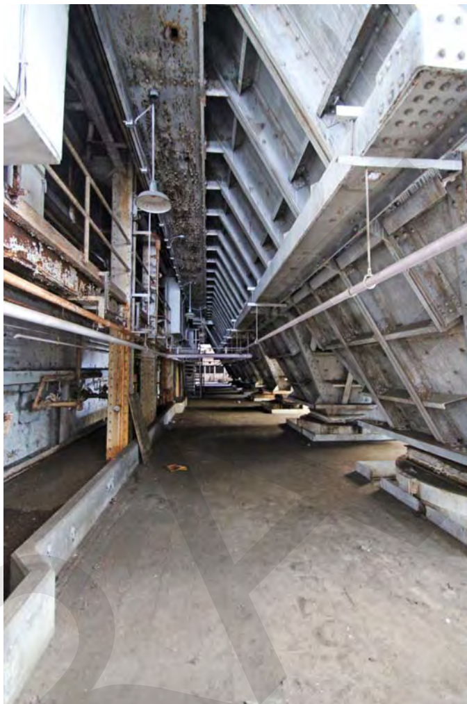
Photo 13- Boiler House interior, typical firing aisle.
