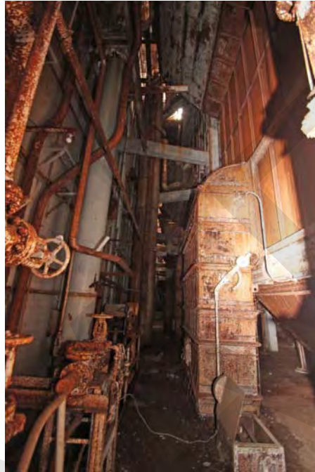
Photo 11 - Boiler House interior, typical boiler equipment.
