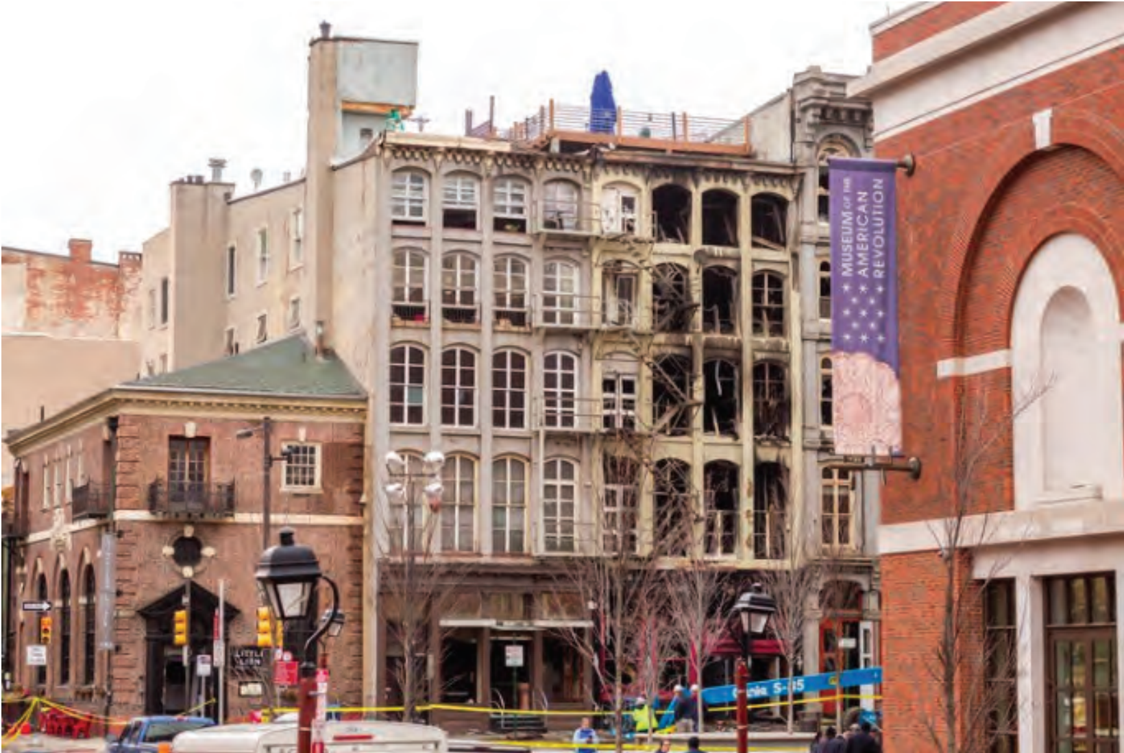
LOCATION A - VIEW FROM 3RD STREET POST FIRE (2018)
