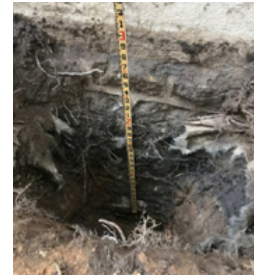
Test Pit TP-2, No Footing Encountered, Geotechnical Report, September 2019
