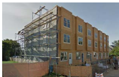
Figure 41: Photo of Townhomes on 100 block of E. Phil Ellena during Construction Phase
